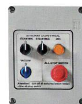
EXTERNAL SWITCH-BOX QUADRO COMANDI
